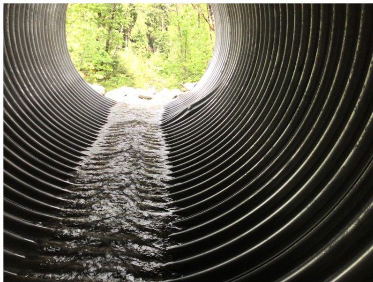
Minor damage noted on floor
